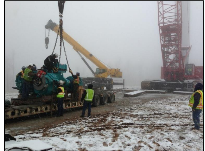
Gear Box, December 2012 Moventas
