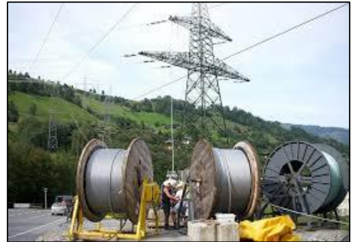
Transmission Cables, July 2011 Iberdrola
